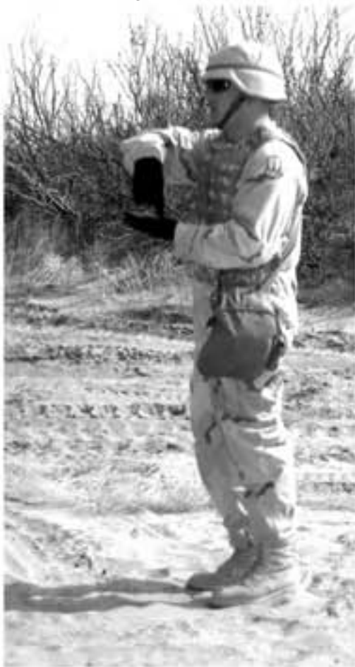
Spc. Jamie Lindsey gives the "cable down" signal to the crane operator.
